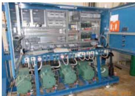
Fig. 2 The CO 2 compressor rack
