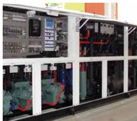
Fig. 5 The refrigeration system
